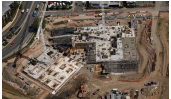
Aerial photograph of Riverpark Building site on 12 February 2009 showing the current status of the works; with two cranes installed and operational, bulk earthworks completed, basement levels substantially completed and works commencing to the ground floor entry level.
